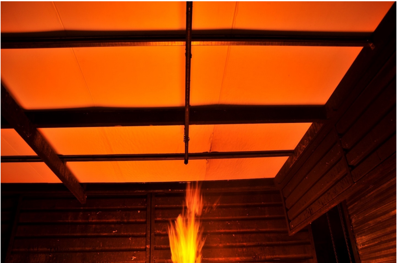
Figure 4.2: Discolouration on joint
