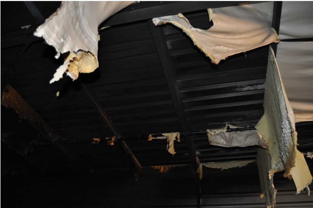
Figure 4.12: Material draped over sprinkler
